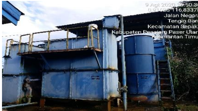
Gambar 5. 9 Instalasi Pengolahan Air PDAM Intake Sepaku
